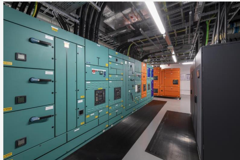
A new £31m wing of the Advanced Computing Facility has been built for the exascale supercomputer
